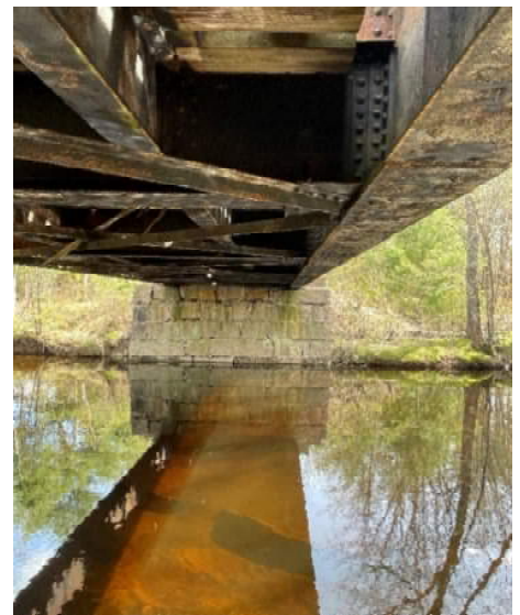
Figure 17: Shepard’s Brook Bridge – Stone Abutment and Bottom of Steel Through Girder Superstructure
