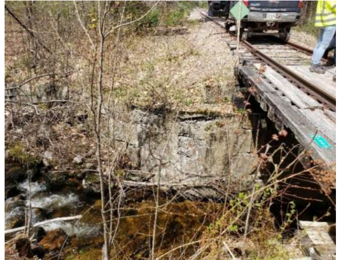
Figure 14: Red Mill Brook Bridge – Concrete Faced Stone Wingwall with Spalling and Undermining Ties
