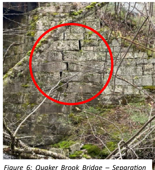
Figure 6: Quaker Brook Bridge – Separation Between Wingwall and Breastwall
