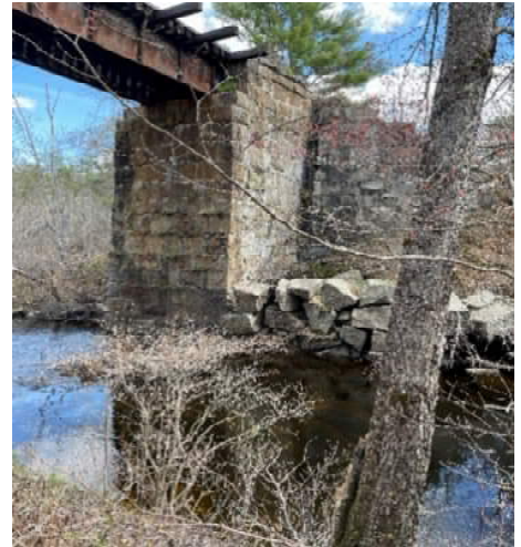
Figure 16: Ten Mile Brook Bridge – Stone Abutment with Return Wingwalls and In-Line Wingwalls
