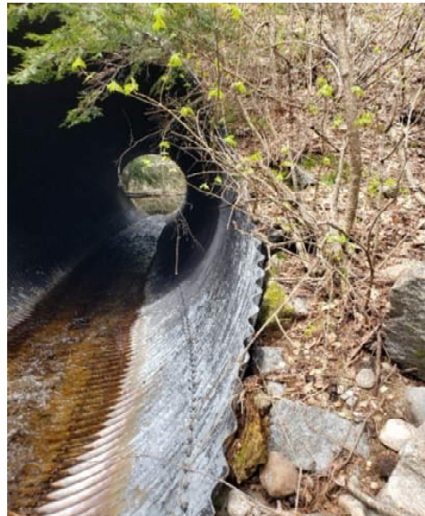
Figure 10: Dug Hill Brook Bridge – Steel Multiplate Culvert with Rust Losses Along Culvert Invert
