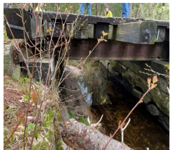
Figure 9: No Name Brook Bridge – Stone Abutment with Timber Seat and Steel Stringers Arch Culvert Barrel
